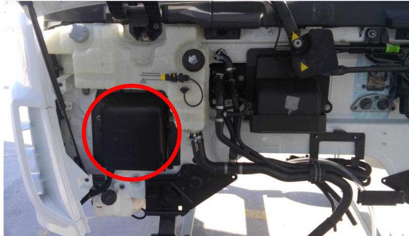
Figure 7-3.1 Electrical Junction Box Location
